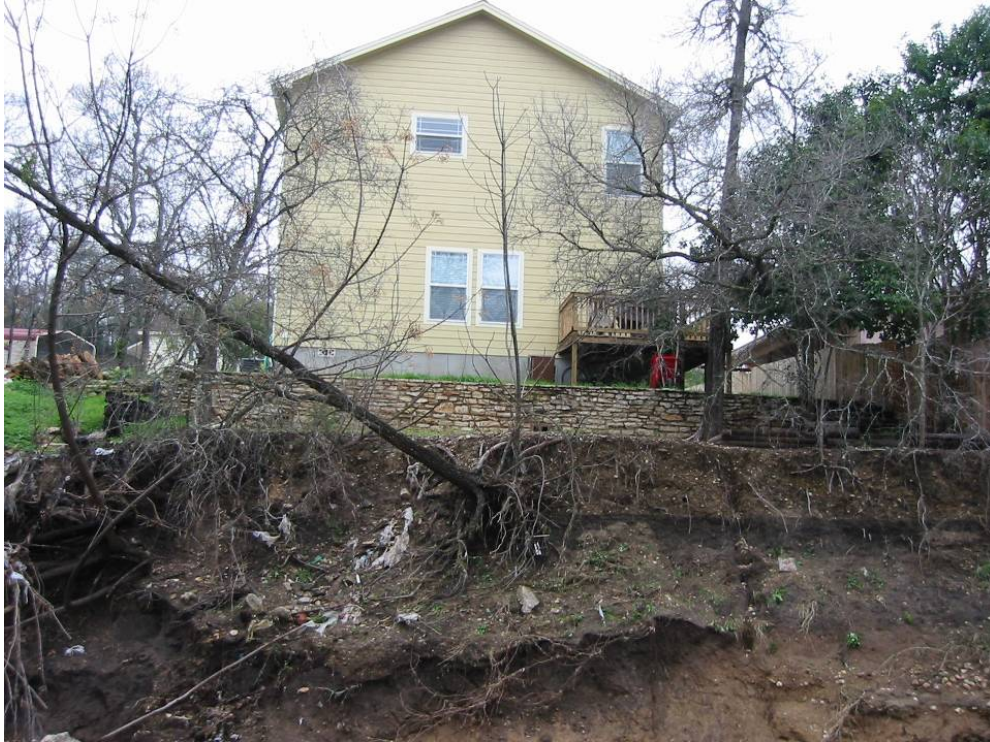
House Built within an Erosion Hazard Zone
