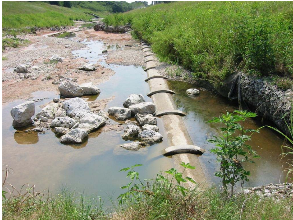
Exposed Utility within an Erosion Hazard Zone
